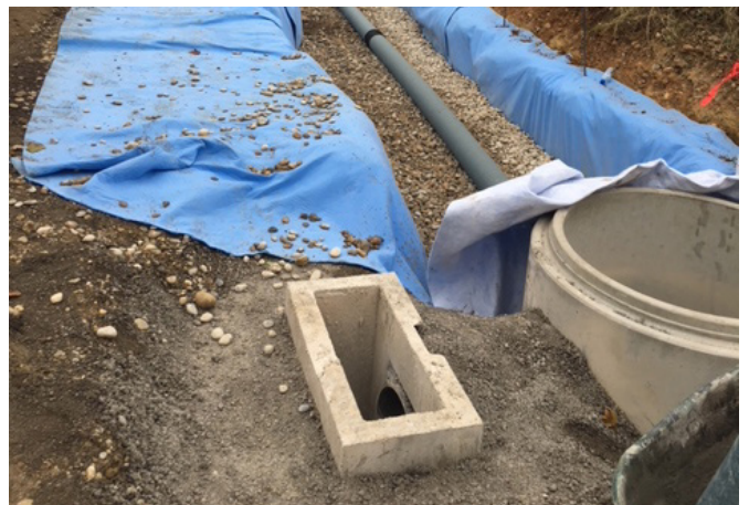
Figure 4: Injection well to collect rainwater on the surface and inject it into the infiltration trench
